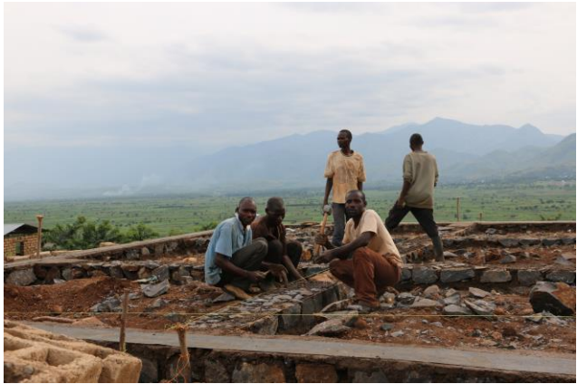
Villagers are being trained in disaster resilient building techniques, Rusizi District, Rwanda, April 2016
